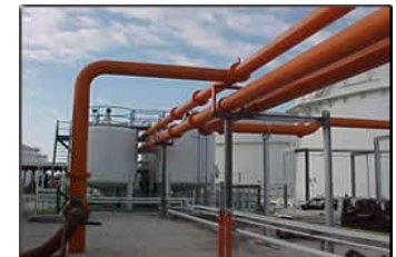
8. Ethanol blended with gasoline (arrived via pipelines) while loading to tank trucks
